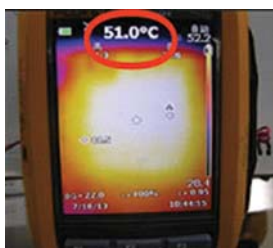
Working temperature on a normal NVR (51°C)
