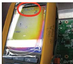
Working temperature on a Uniview NVR (38,9°C)
